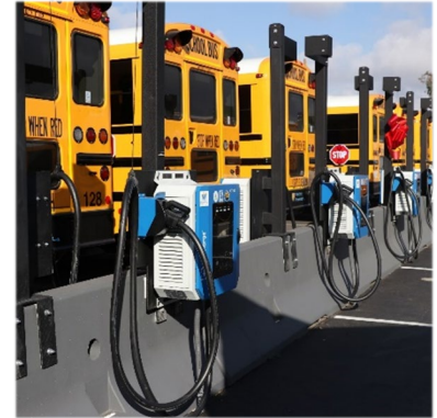
Moreno Valley Unified School District (Moreno Valley, California) electric vehicle fleet and charging infrastructure is designed to meet the district's school transportation needs, reduce greenhouse gas emissions, and improve air quality.
